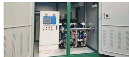
Temporary Water Supply
